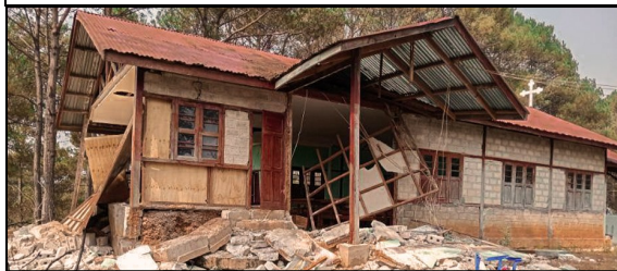
A church in Myanmar damaged by last month's devastating earthquake
